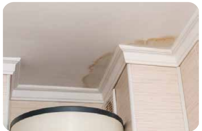
Damp caused by leak
